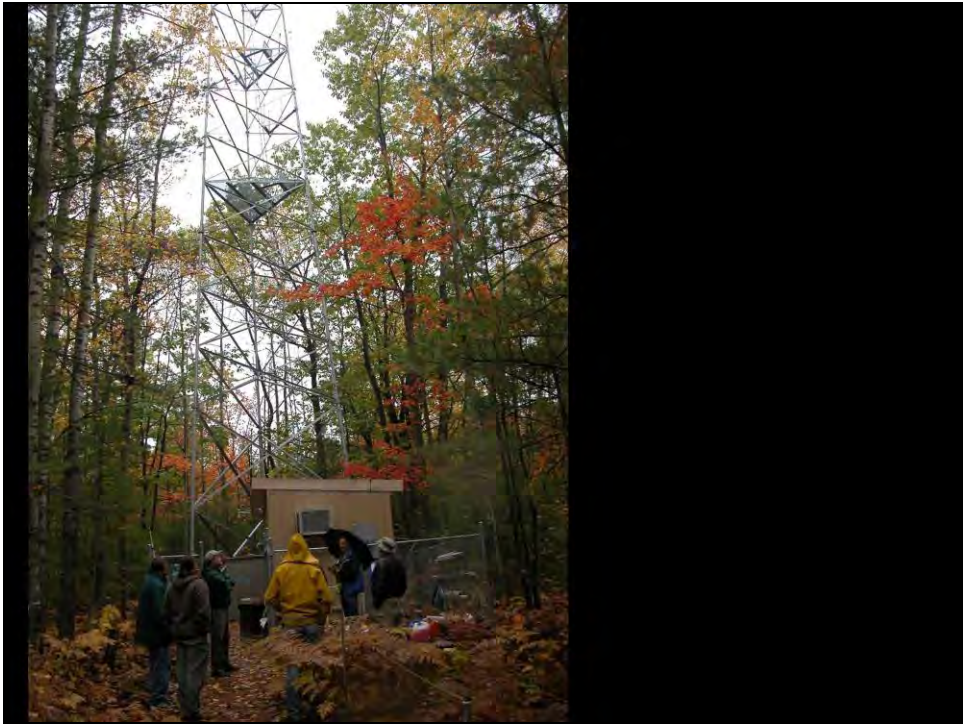
Pipes and wires lead from the instruments on the tower
